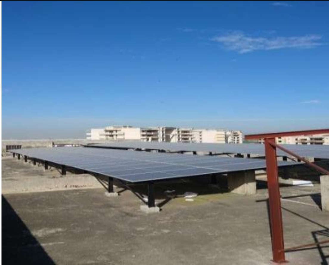
Solar System, Chak Shahzad Campus, Islamabad
